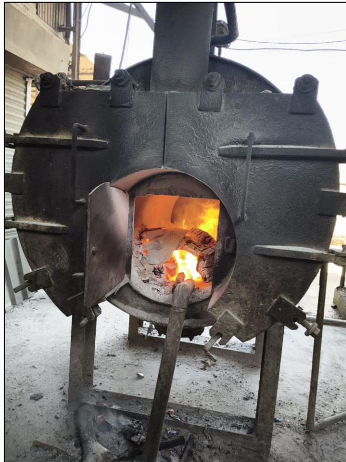
Boiler for Steam Production
